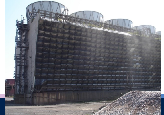
Mechanical-Draft Cooling Tower. Source: Tetra Tech
